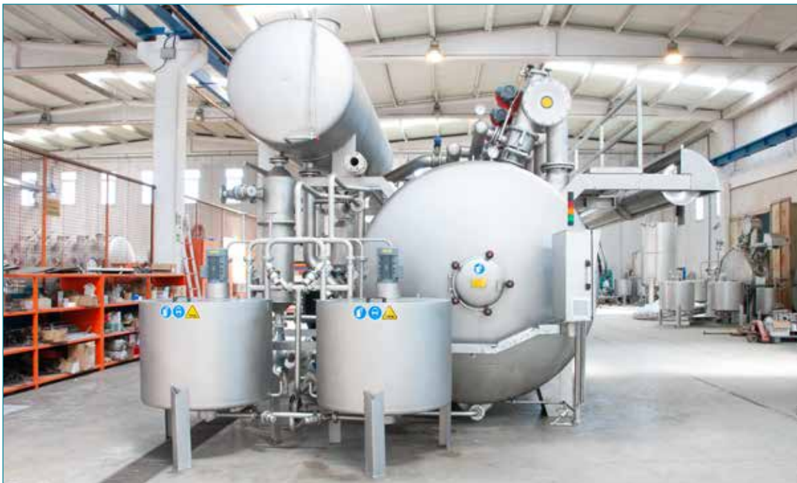
Tam otomatik kimyasal ve boya ilave tankları Fully automatic chemical and dye addition tanks
